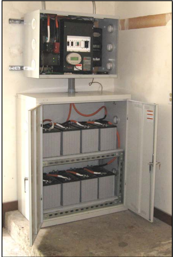
Example of battery back-up system.
