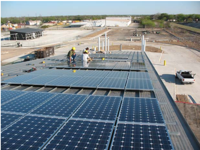
10.5 kW system, South Central Transit & Training Center, San Antonio, Texas
