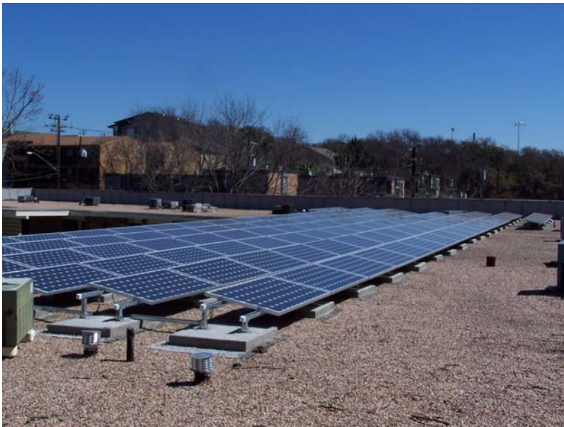
23 kW system, Alori Properties, 3212 Red River, Austin, Texas
