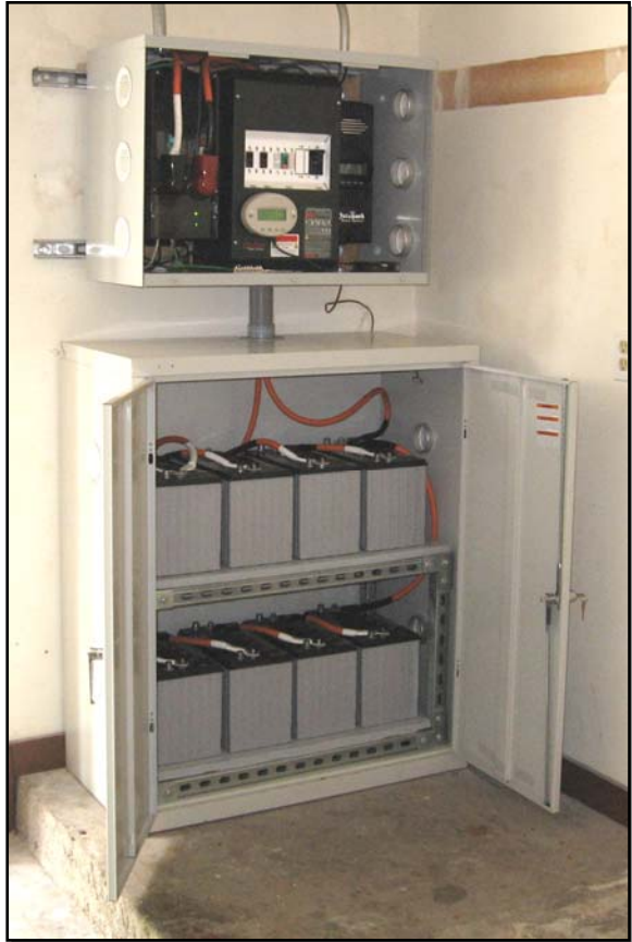
Example of battery back-up system.
