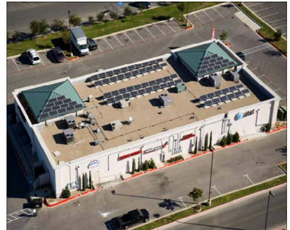
14kW installation at Alori Properties retail center Five Oaks Plaza, 13000 N. IH 35
