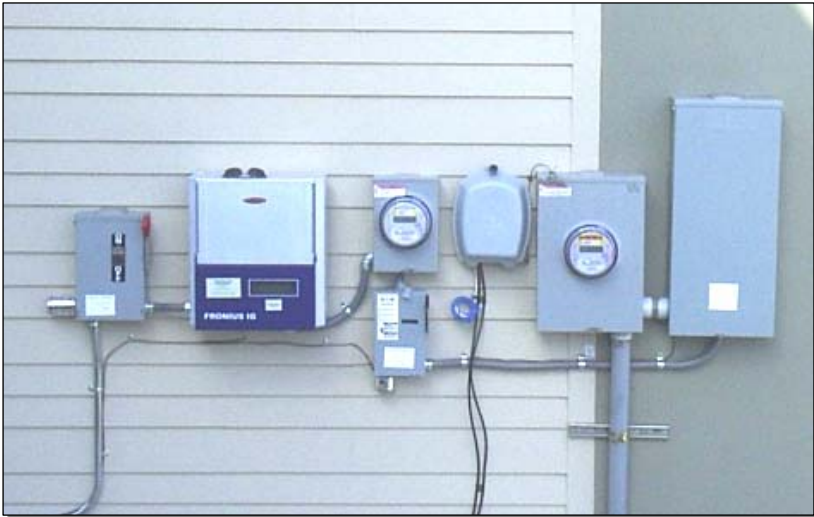
Example of components used to tie into your standard power grid. These will be added (l to r): 1. DC Disconnect 2. Inverter 3. PV Meter 4. AC Disconnect These are pre-existing on your home: 1. Cable/phone box (perhaps) 2. Revenue Meter 3. Breaker Box, or Load Center
